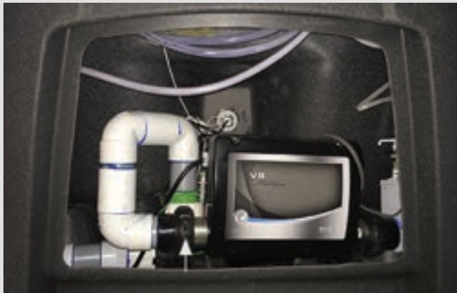
FIGURE 1.9a : HEATER UNION; LOOSEN UP TO BLEED AIR
